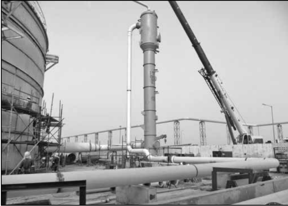
De-gassing Boot erected at a project site in Rajasthan
